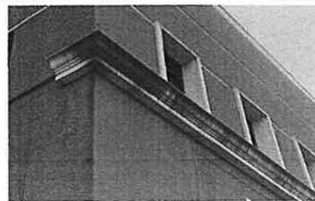
Severe Staining and Water Intrusion in EIFS
