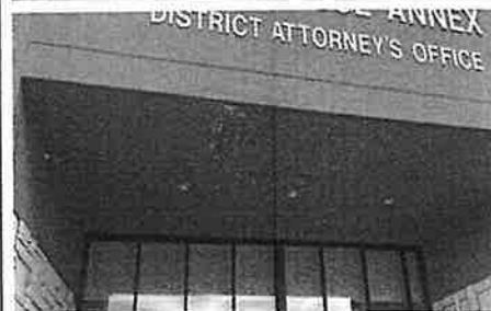
Soffit is Falling at Entrance
